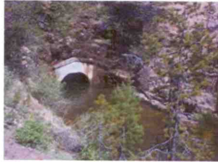
The outlet of the Duchesne Tunnel near SR 150. Water diverted from the North Fork of the Duchesne River is conveyed by the transmountain tunnel to the Provo River, then stored in Deer Creek Reservoir.
