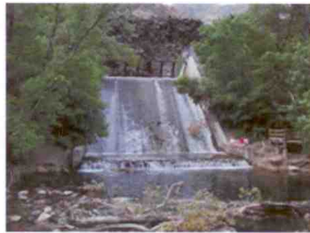
Big Cottonwood Creek as it flows over Utah Power's overflow structure located in the Storm Mountain Picnic Area.
